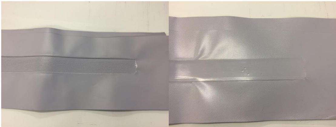
Picture 1. Welded joint of tunnel membrane Protan 514-940, front side to the left and back side on the right.
